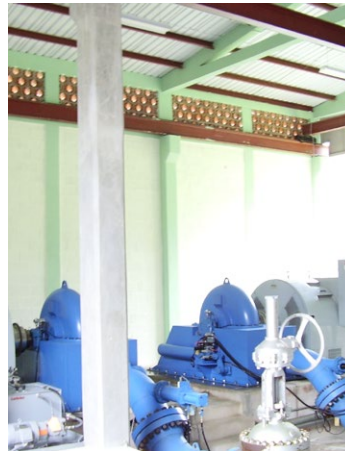
Export System Energy Recovery (photo courtesy of Canyon Hydro)
