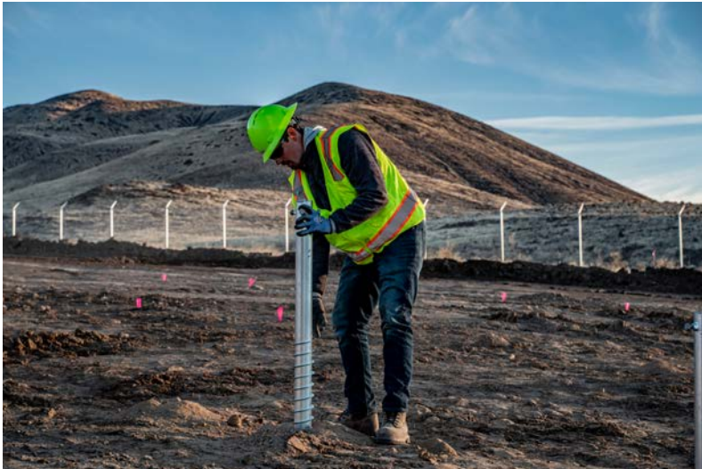
Figure 2-2. Photographic Examples of the Solar Arrays and Foundation
