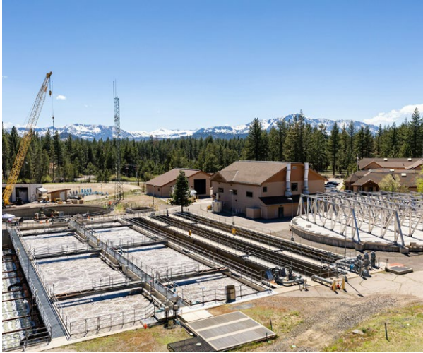
STPUD Wastewater Treatment Plant
