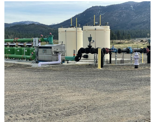
Recycled Water Distribution Infrastructure
